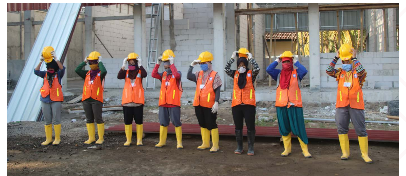
A photograph taken in 2019 shows construction workers putting on protective equipment at the site of a PETRA initiative to rebuild Palu, Central Sulawesi, after the 2018 earthquake and tsunami. ©UNDP
